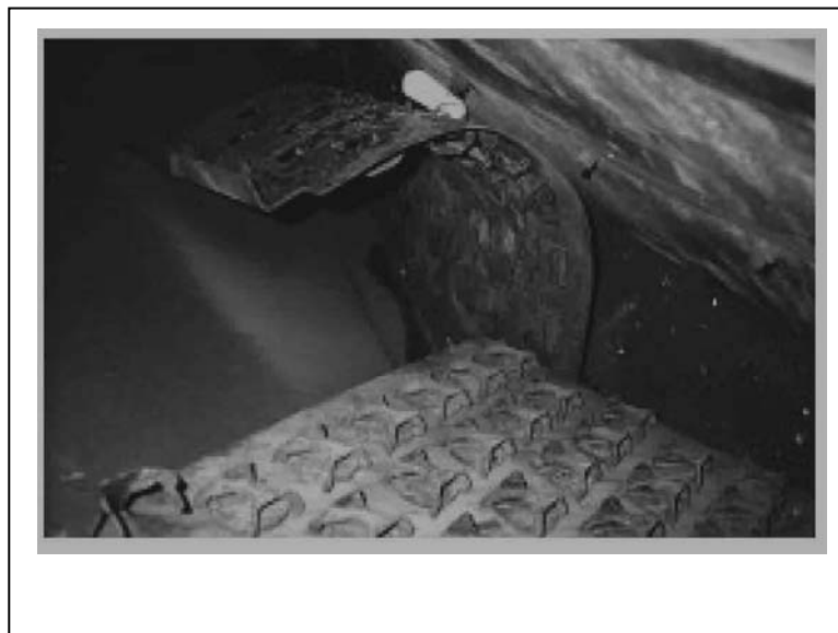
Fig.2. Stripping and wash section tray damage .
