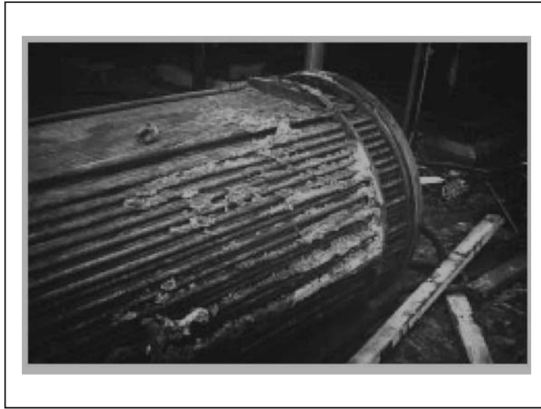
Fig.3. Fouled overhead exchanger bundle.
