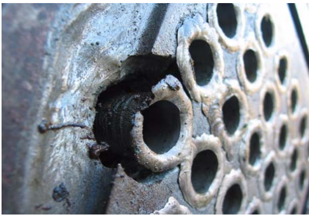
Failure for the seal welding of the tube to tubesheet
