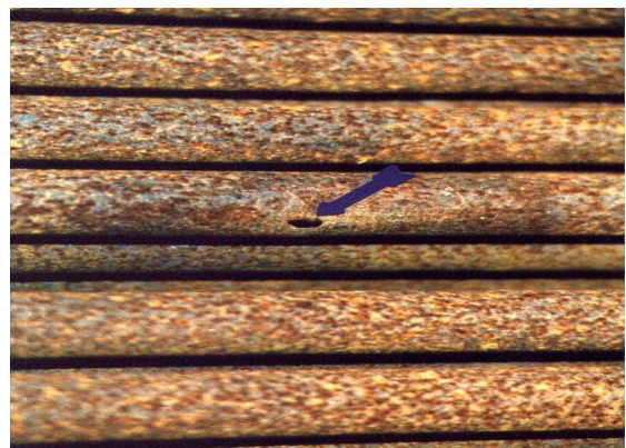
Localized Corrosion and pitting
