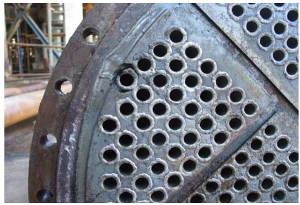
M-EA507 Tubesheet Layout – shows the location of the failed tube to tube sheet.
