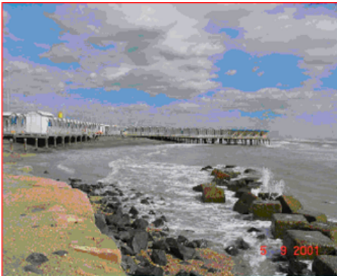
Figure 9 - Section 2: South “Vecchia Pineta” 7 months after BMS construction (BMS broken)
